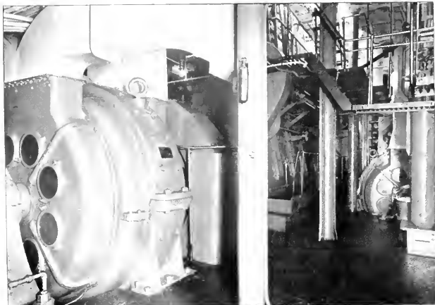
An excellent example of the adaptability of the diesel-electric plant to marine uses is found in its application on hydraulic dredges. The illustration herewith is a view in the engine room of one of the U. S. Army dredges recently completed. It shows one of the McIntosh & Seymour-Westinghouse diesel-electric generators, of which there are four on each dredge, supplying power for the dredge pumps, a propelling motor, and all of the auxiliary machinery.
